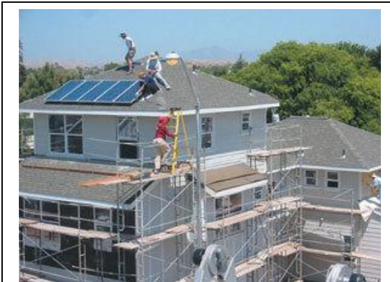
Installing solar panels on the new East Bay houses HABITAT FOR HUMANITY
