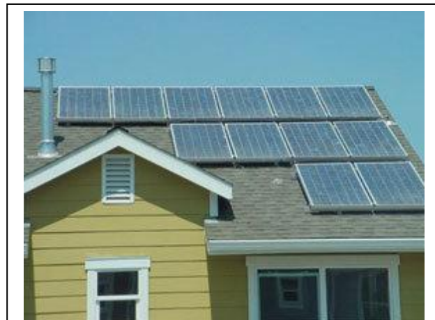
The solar panels on the Livermore estate were provided by Powerlight HABITAT FOR HUMANITY
